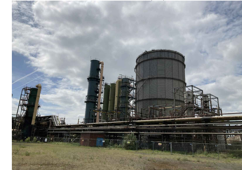
BENZOLE TANKS AND ASSOCIATED PLANT
